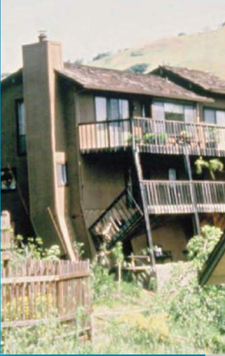
The balcony of this hillside home partially collapsed and the home tilted when the stilt-type support posts and poorly braced walls shifted during an earthquake.
