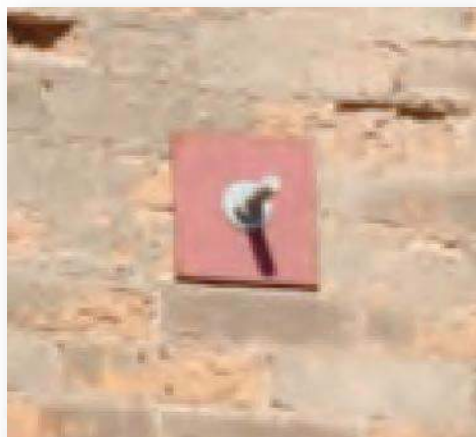
A steel plate with anchor bolts.
