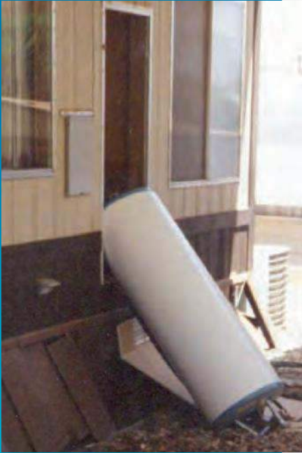
During an earthquake, an unbraced water heater can topple, which can start a fire or lead to major water damage.
